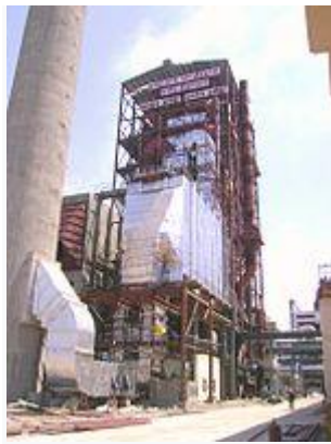
Chemical recovery boiler at Pugalur
