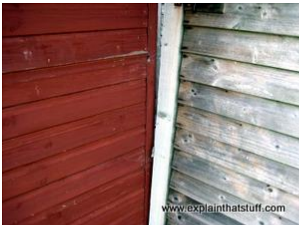
Photo: A fence before (right) and after (left) treatment with wood preservative.
